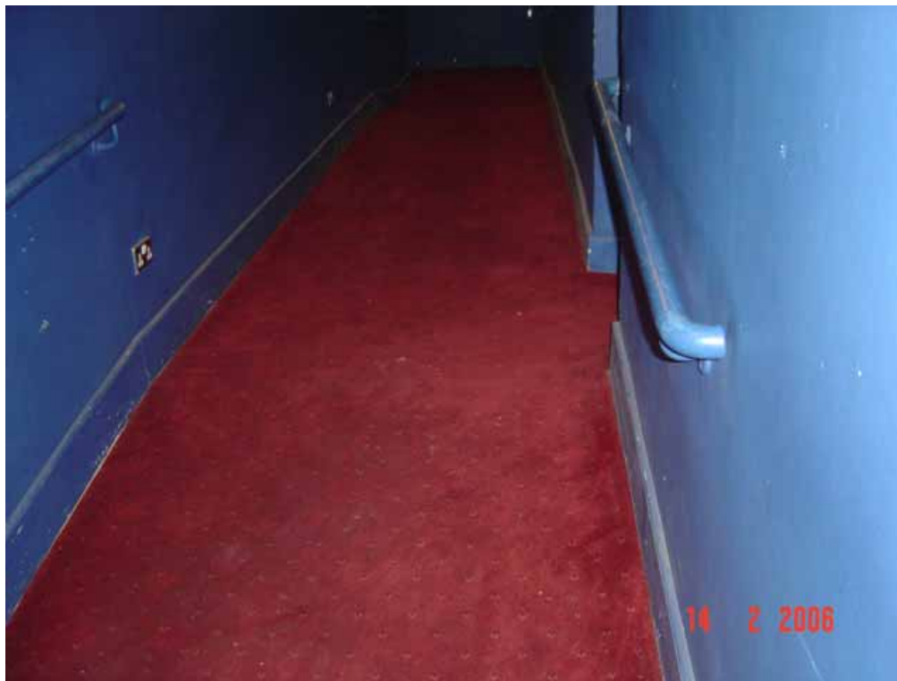
Fig 7.5 Ramp section with handrails but unfortunately to tactile hazard warnings at the top or bottom
