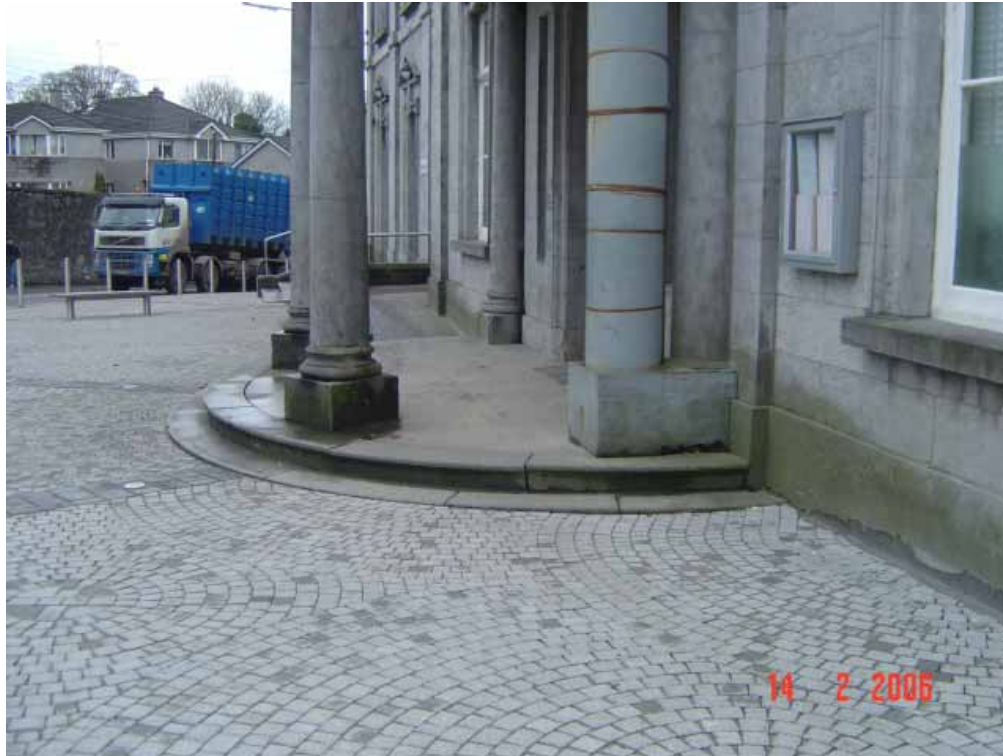
Fig 7.4 These steps have no tactile hazard strips plus the steps have no visual contrasting from the surrounding area
