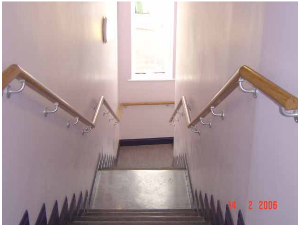
Fig 5.2 Stairs down from library showing good handrails but no tactile warnings.
