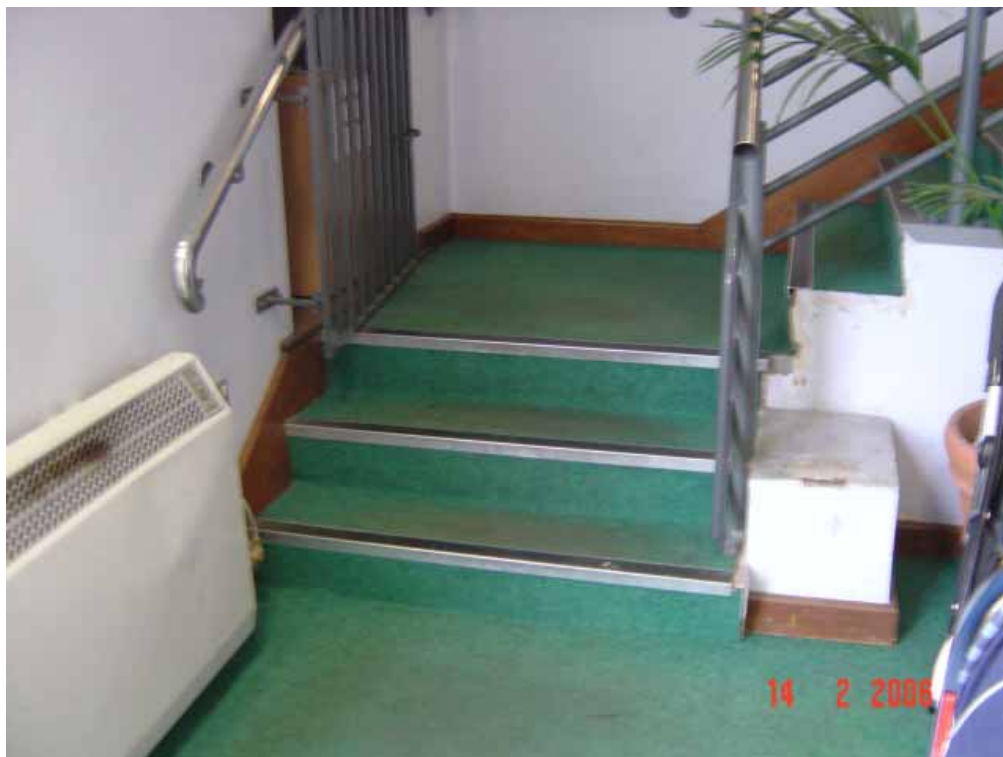
Fig 9.2 These steps make access to this office impossible for a person in a wheelchair.
