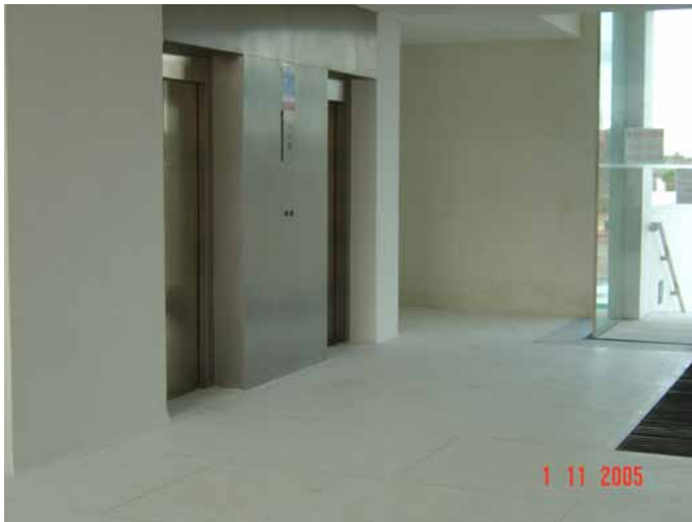
Fig. 1.3 No tactile warning outside lifts
